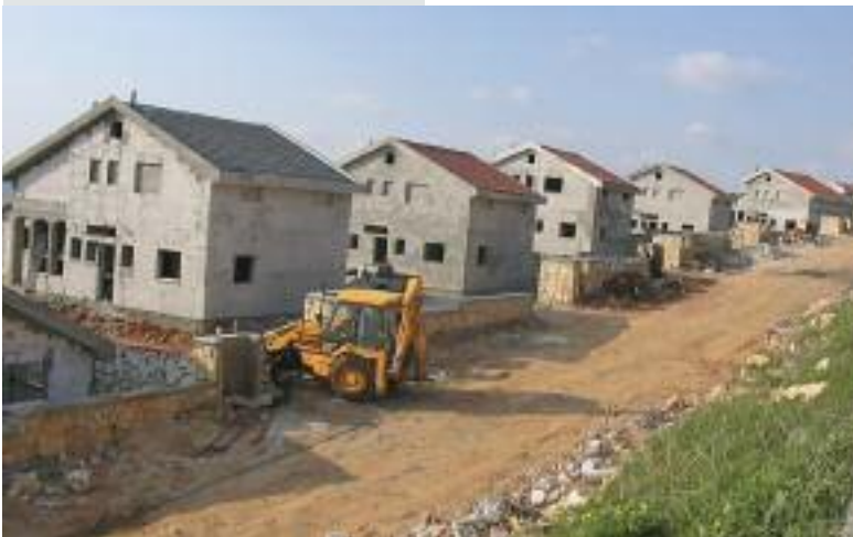
New houses in the Revava Israeli settlement which are being built on Palestinian land confiscated from the nearby Hares and Deir Ballut villages in the West Bank
