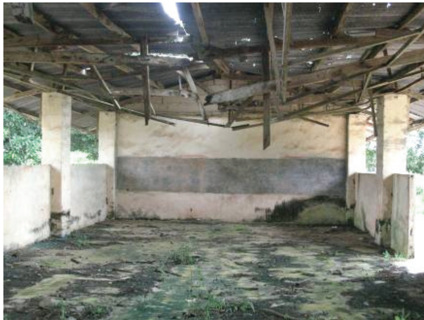
A primary school in Khana local government, Rivers State. This classroom was abandoned after the roof nearly collapsed, forcing students to cram into the sole remaining classroom or learn outside. © 2006 Chris Albin-Lackey/Human Rights Watch
